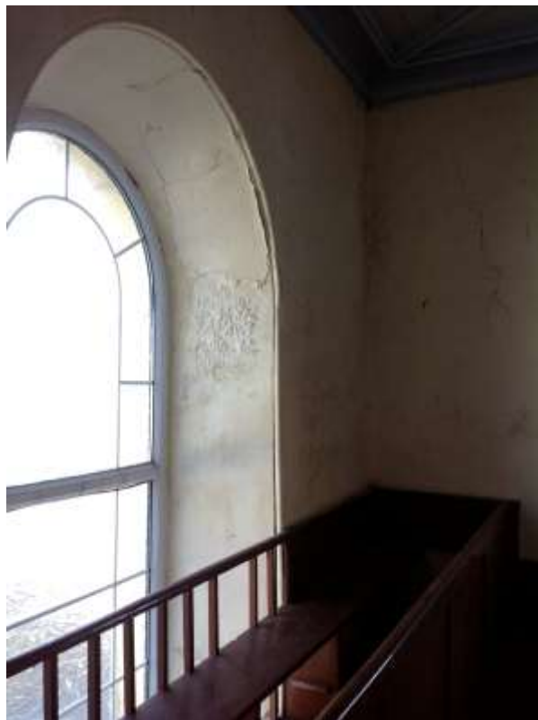
Defective internal finishes to window areas.
