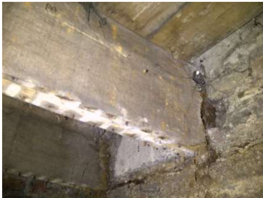
Decayed timber joist end
