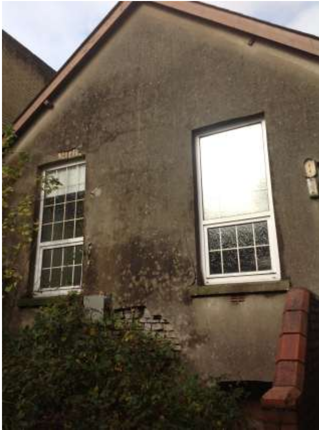
Defective render & wall to rear of kitchen. Joist ends have rotted.
