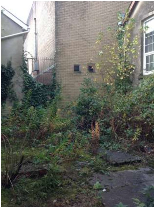
Overgrowth to rear garden
