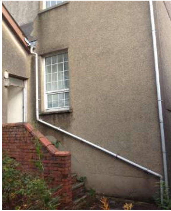
Missing gutter end cap and defective pointing to wall. Steps are uneven
