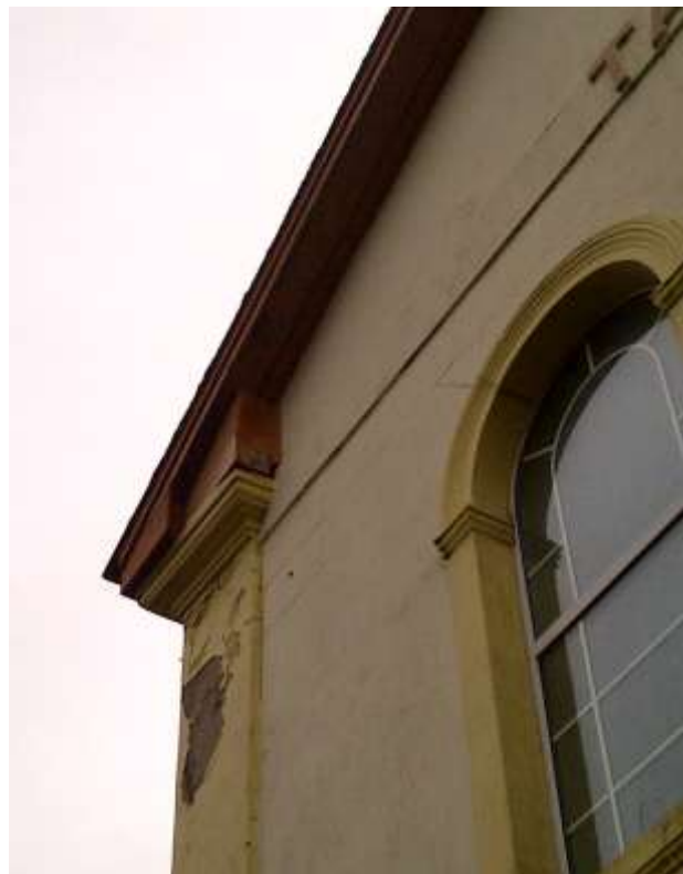
Front wall with water damage from missing gutter section
