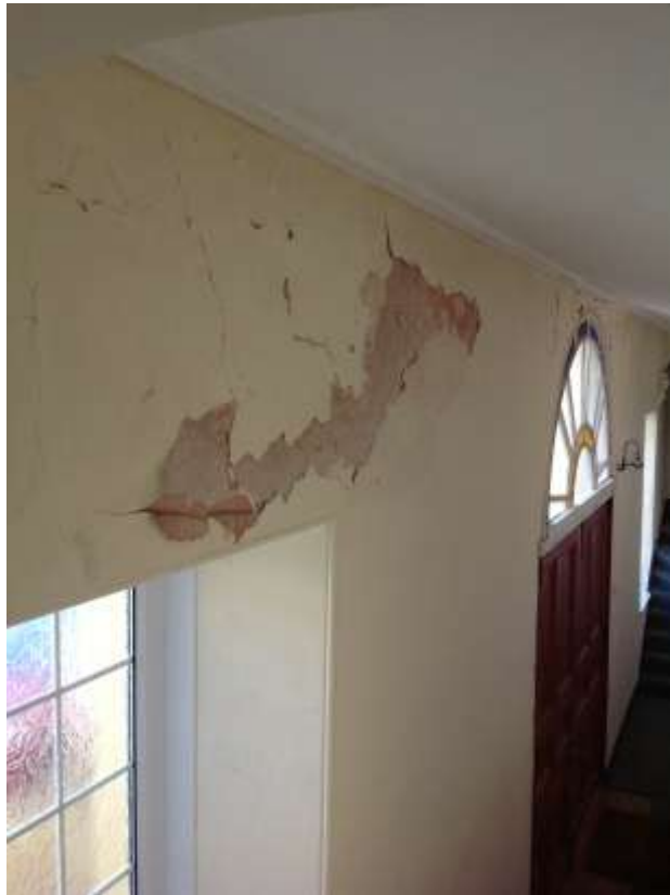
Internal finishes effected by damp
